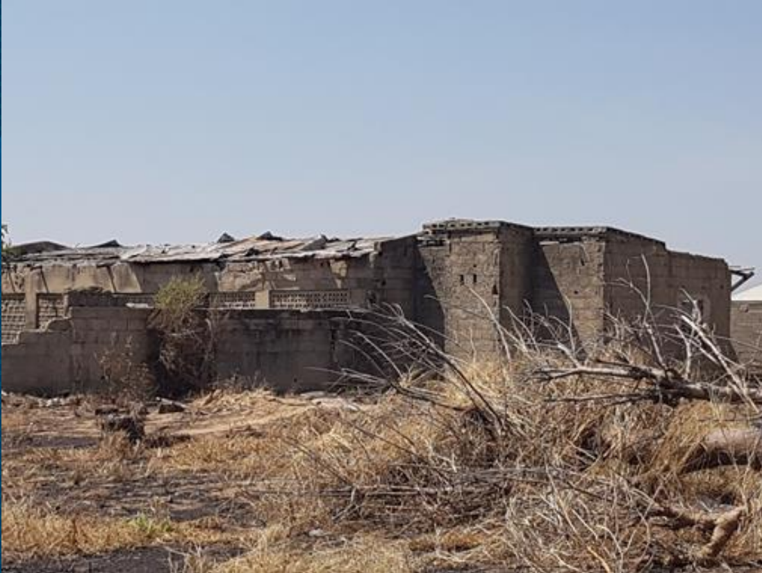
A destroyed house after the attack (Photo: UNDP Nigeria)
